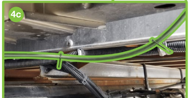
The photos above show Cable 2 being routed and secured along the bottom of the cab. Preexisting tie mounts provide secure many mounting points.
