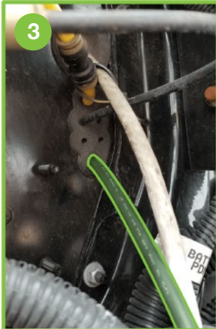
The image above shows Cable 2 coming out of the firewall grommet and into the engine bay.
